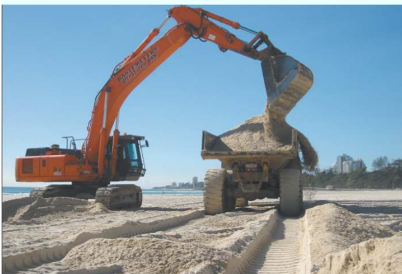
WORK is continuing on the removal of 100,000 cubic metres of sand to restore the once famous Kirra Point
